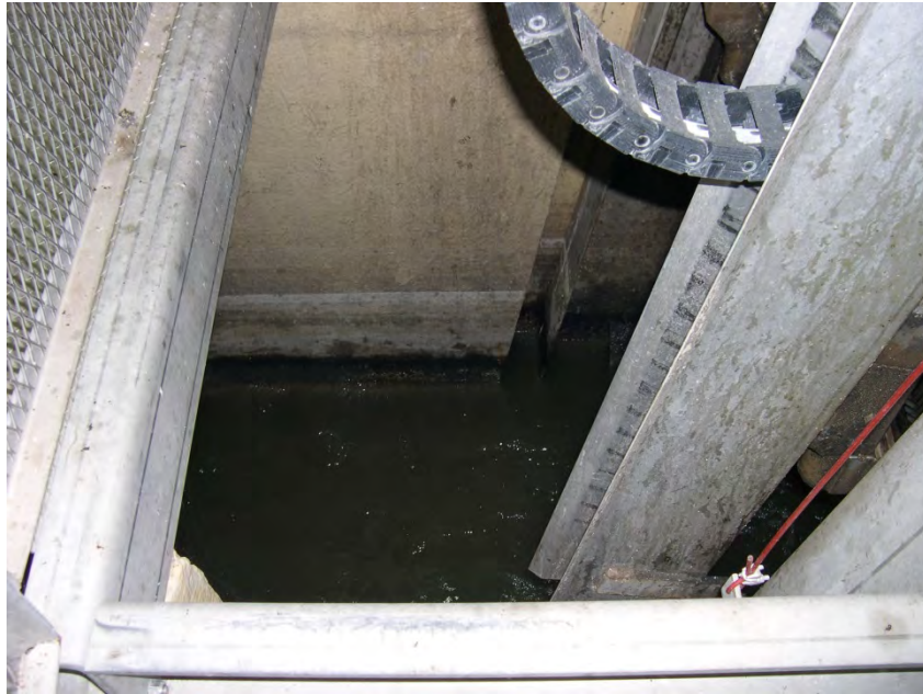
Sewage tank. Photo: EF
